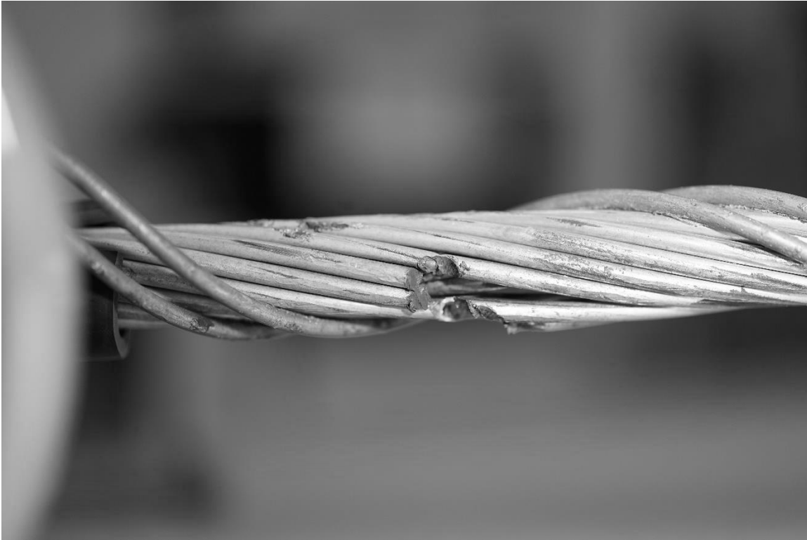
Figure 31. Electrical arcing on the center phase conductor.
