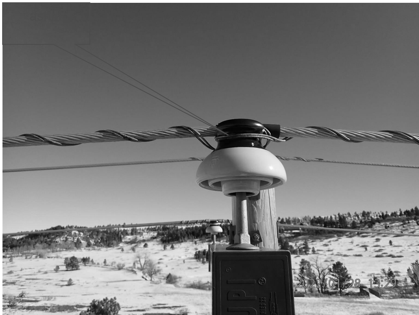
Figure 19. West phase pin insulator.
